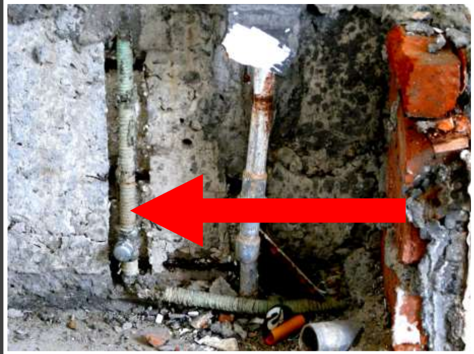
Rope Lagging 熱水喉隔熱石棉繩
