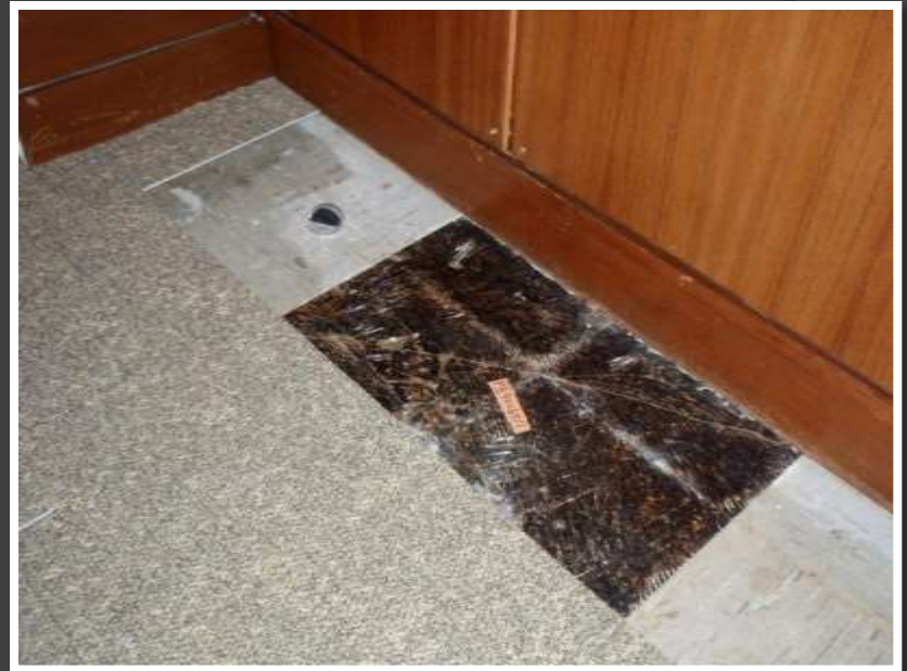
Vinyl Floor Tiles 含石棉的膠地板
